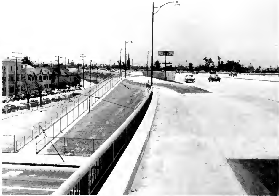
Looking southerly along completed section of Harbor Freeway from above Pico Boulevard, showing bus turnout on east side of freeway for northbound traffic. The city street shown on extreme left is Bond Street.
